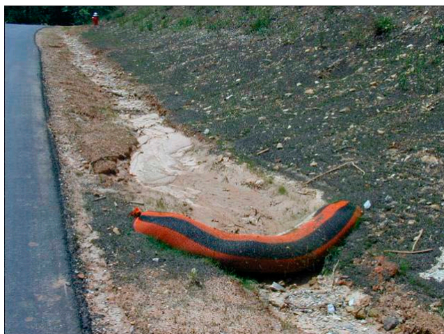
Figure 3 Compost filter sock check dam
