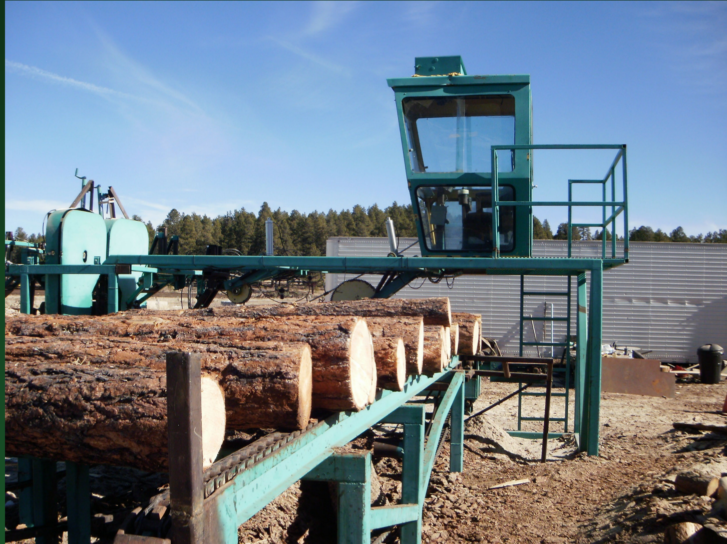
Small-Diameter Ponderosa Pine Log Processing Facility in Northern Arizona. Image Source: USDA Forest Service
