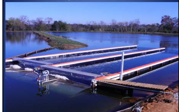
Completed unit with WW units in place and operating. Units are 16' by 80', 4 feet operating depth. Wall tops are wooden and painted orange with sand mixed into the paint to afford assess.
