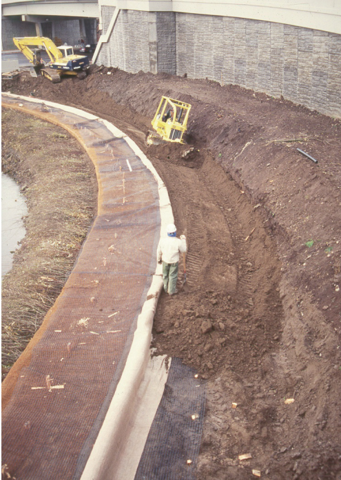
Figure TS14I-30 Fill placement within VRSS ( Photo courtesy of Robbin B. Sotir & Associates, Inc. )
