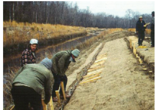
Figure TS14I-19 Installation of live fascines combined with erosion control fabric ( Photo courtesy of Robbin B. Sotir & Associates, Inc. )
