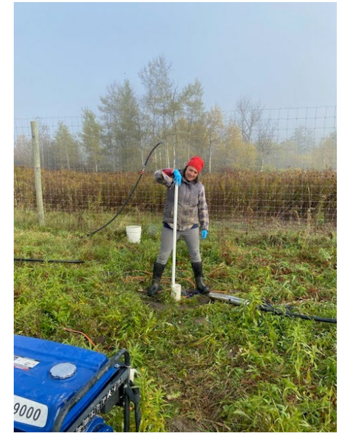
"Plunge" along and above the well screen
