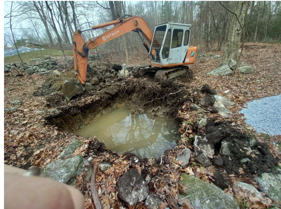
A well installed too shallow.
