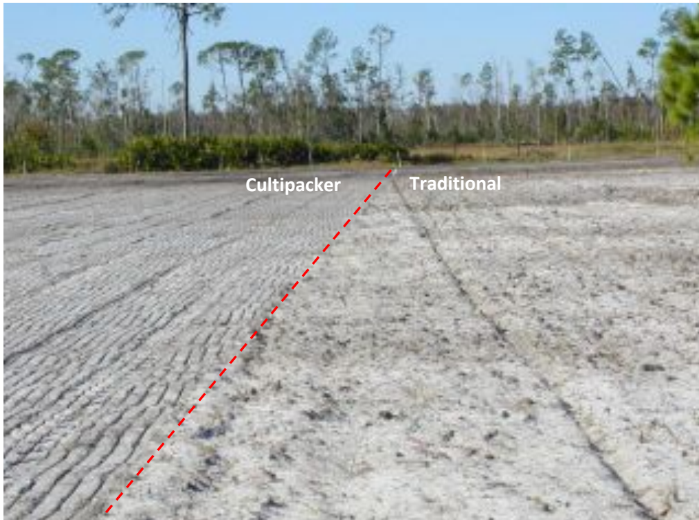
Figure 9. Hilochee WMA groundcover restoration site showing soil compacting using a cultipacker on half of the area (left side of photo), and a traditional roller compactor on the other half (right side of photo).
